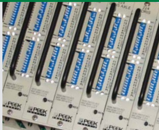
Peek SmartToll installed in new AETC system
